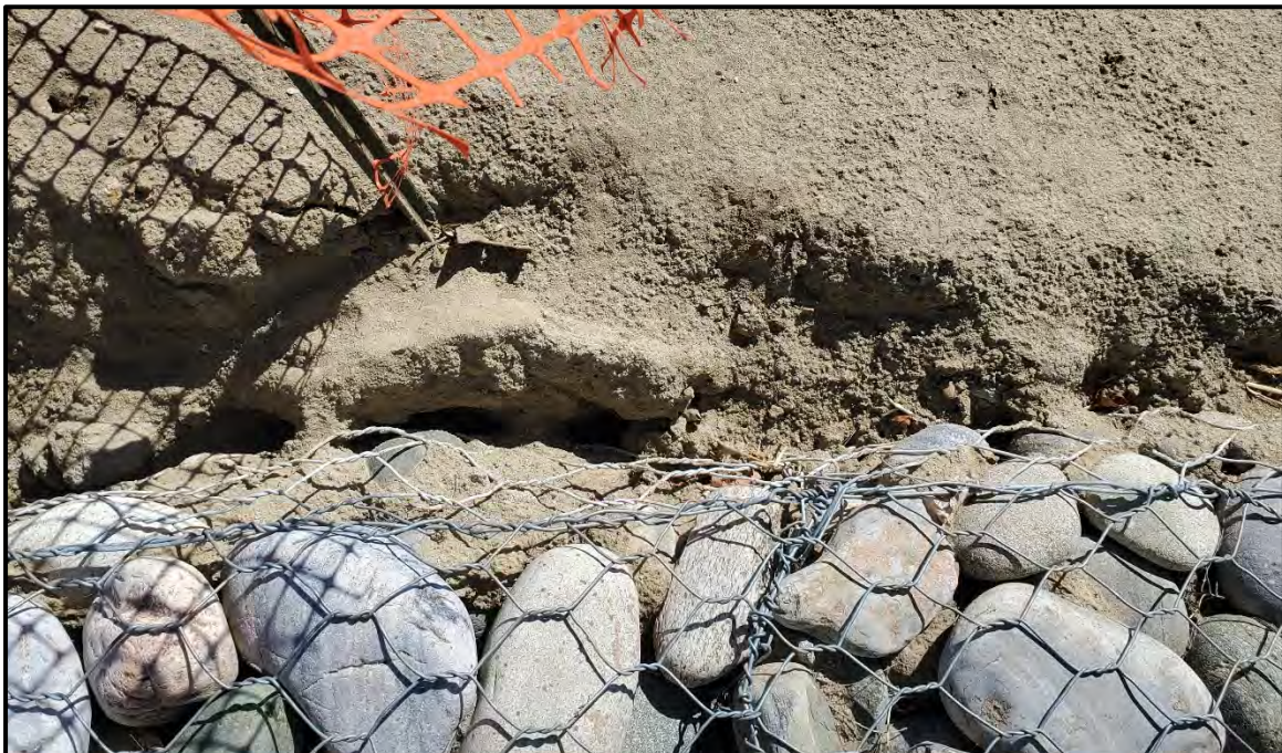
Piping behind Damaged Gabion Wall near Boring B-3 View Towards the East
